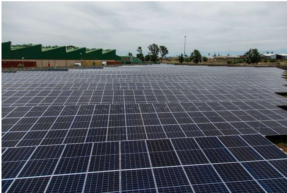
Henkel South Africa unveils 100% sustainable Alrode plant with solar farm installation.
