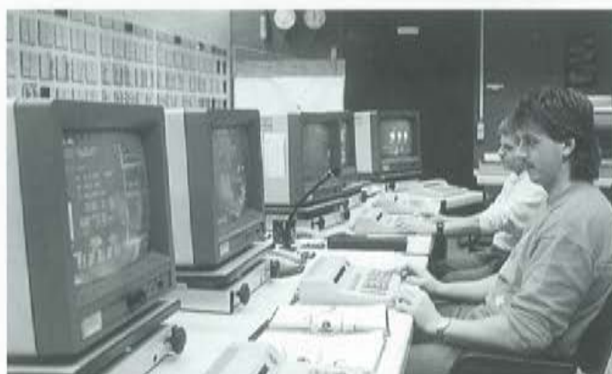
Computerized process control: a modern control room in the adhesives plant.
