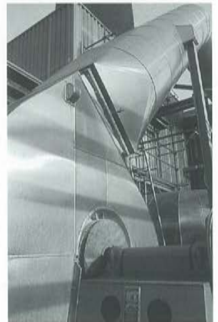
Reducing emissions by means of newly developed plant and processes: part of Henkel's power station at the Düsseldorf parent plant.
