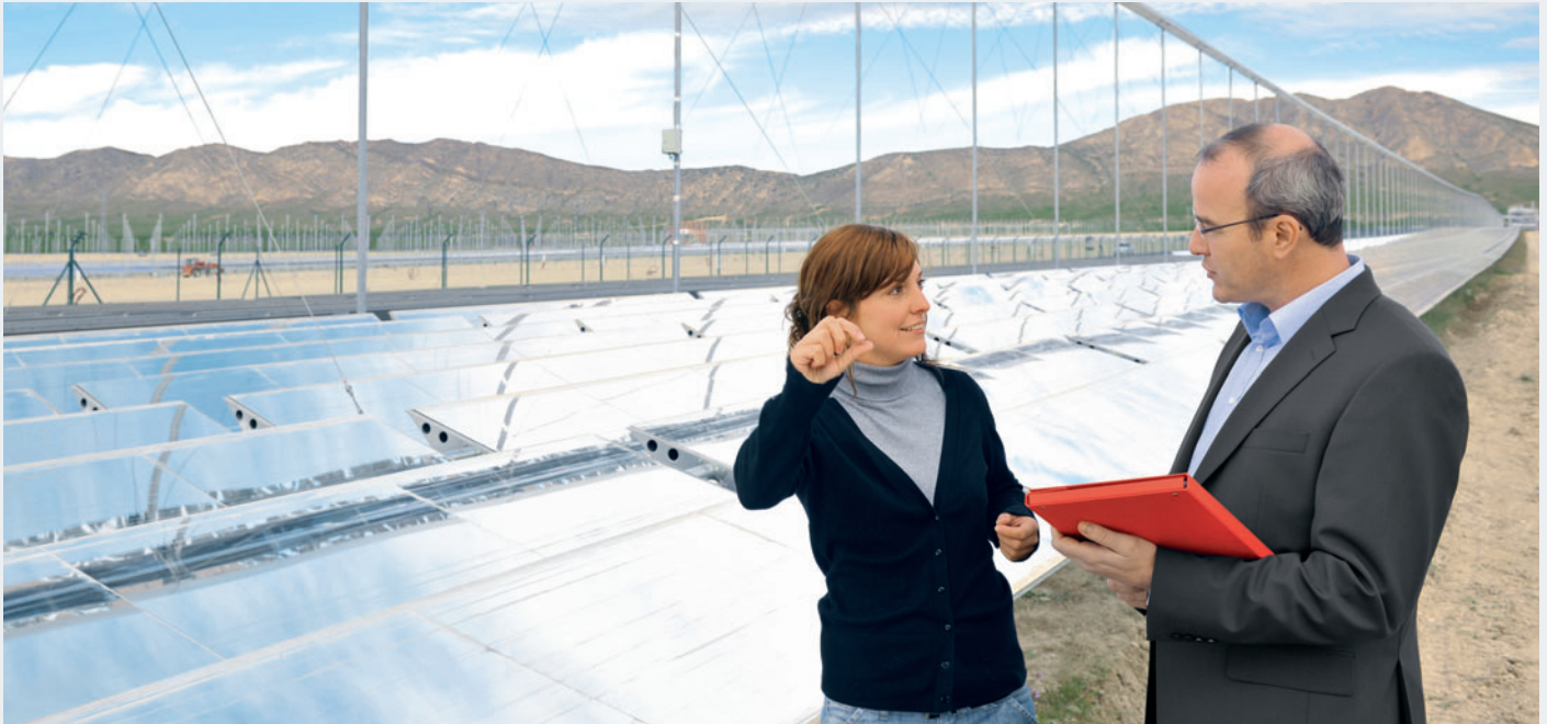
Puerto Errado 1, the pilot solar thermal power plant of Novatec Biosol, is located in Southern Spain. Meike Schumann, quality engineer at Novatec Biosol, and Thomas Wittmann, field representative at Henkel, discuss the performance of Henkel's Terostat MS adhesive right at the plant.
