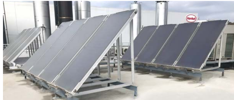
The hot water at our new plant in Gebkim, Turkey, is generated using solar energy.
