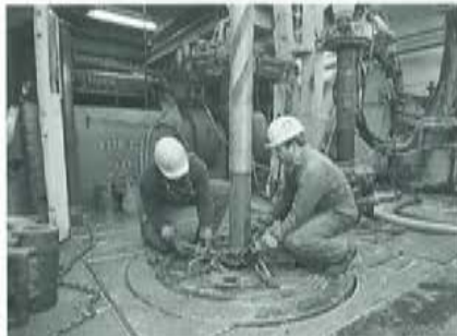
A drill rod being extended on a drilling platform. Counter-rotating multiple toothed cones enable the drill heads to eat through the most stubborn rock.
