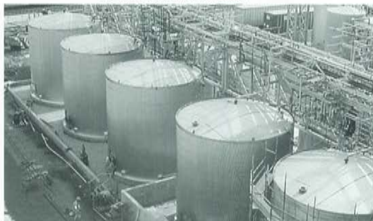
The Henkel subsidiary in the USA produces 25,000 metric tons of alkyl polyglycosides per year. The plant in Cincinnati, Ohio, is the biggest of its kind in the world.
