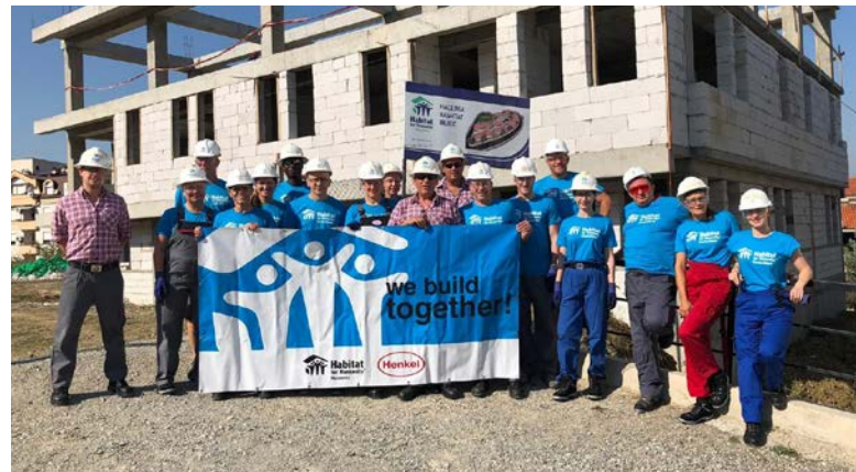
Henkel employees, together with the Habitat for Humanity organization, help to provide families with a new home by going on building trips like this one in North Macedonia.
