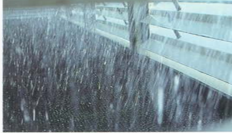
Noise prevention in Düsseldorf – drip impact attenuators reduce water noise in a cooling tower.
