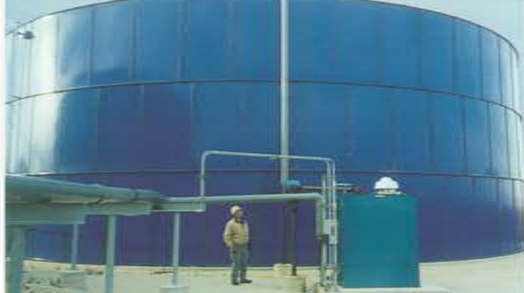
Odors can no longer escape from Henkel Corporation's wastewater purification plant in Kankakee. The new equalization tank is shown here.
