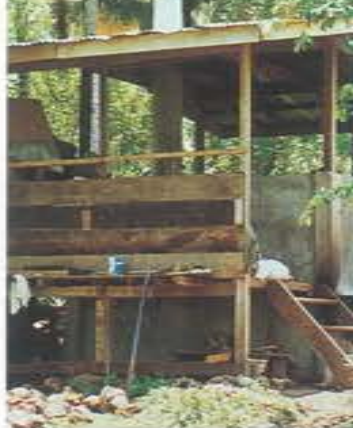
The social project for Philippine coconut farmers is making good progress. Henkel helps to finance the construction of copra dryers.
