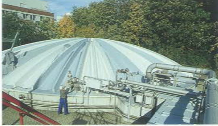
Henkel in Düsseldorf-Holthausen has considerably reduced its wastewater volume and AOX load. The central wastewater monitoring plant is shown here.
