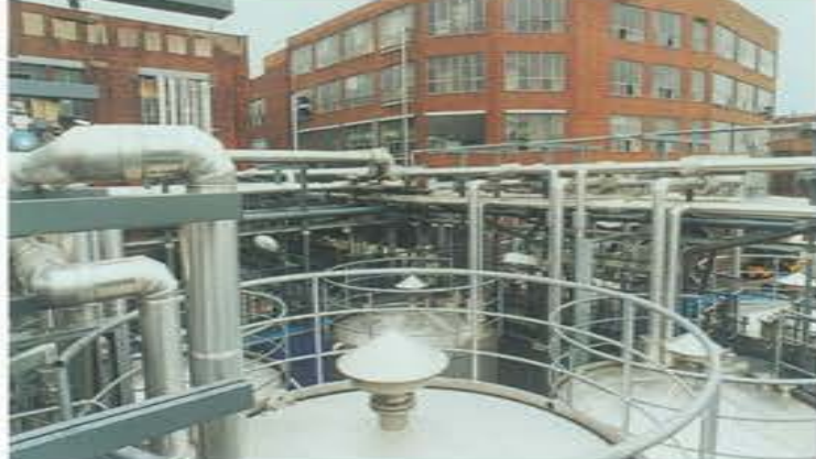
Environmental protection is also a top priority at Thompson-Siegel in Düsseldorf. The tank farm can be seen in the foreground.
