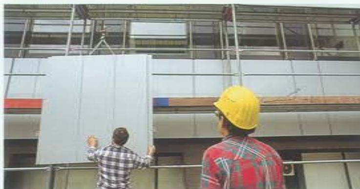
World premiere at Henkel in Düsseldorf – the first building with façade and windows made from chrome-free pretreated and coated aluminum.
