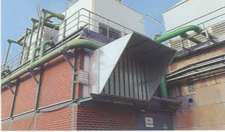
Lower noise emissions from a sulfation plant in Düsseldorf, thanks to noise dampers, which have been fitted to the ventilation gratings of a room that houses large and noisy compressors.
